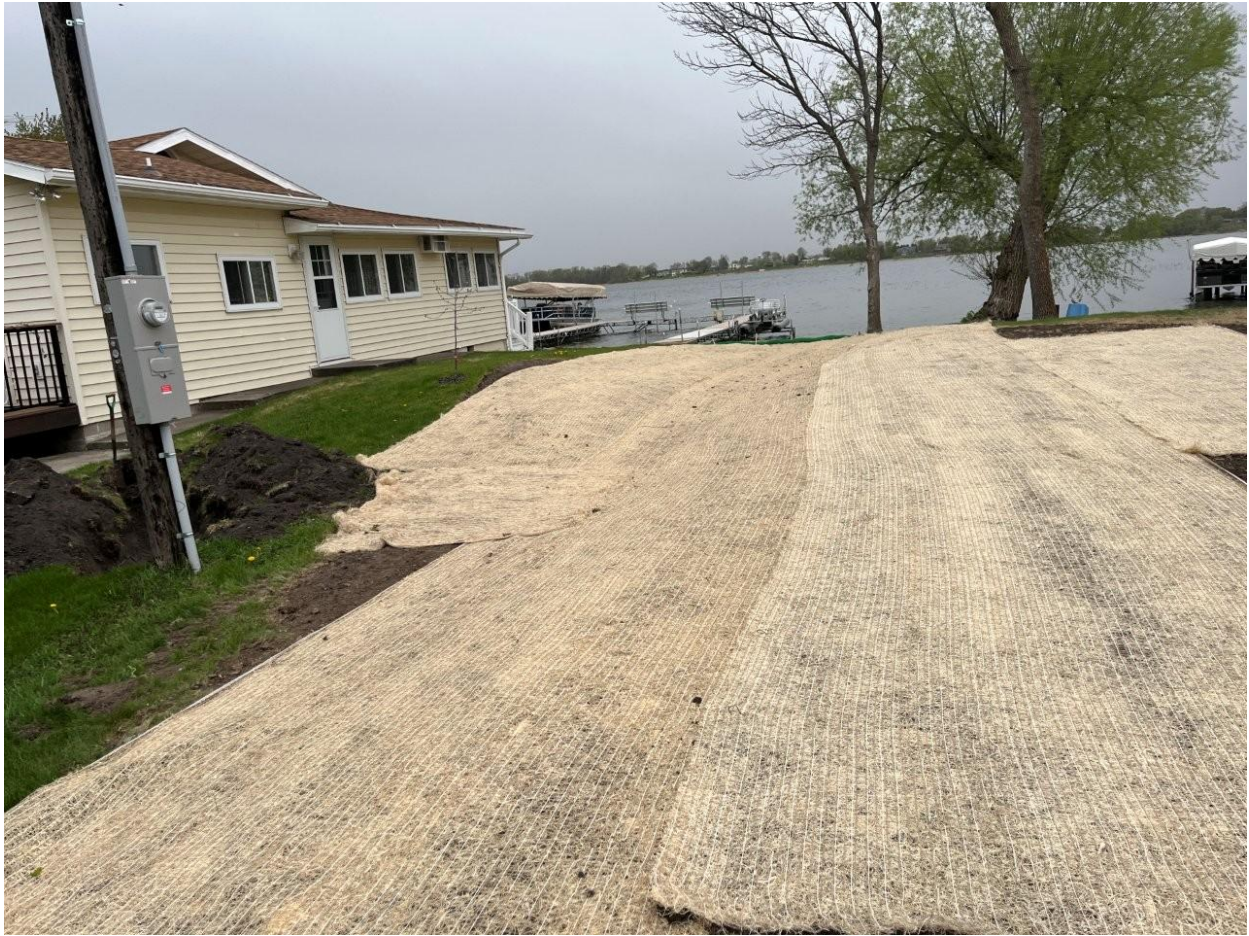
Constructed waterway which allows for a stable drainage area down to the lake when the catch basin gets overwhelmed during large rains events.
