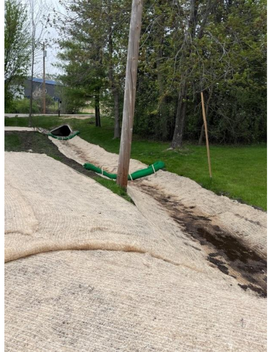
After – Accumulated Sediment removed from ditch and side slopes stabilized with erosion blanket.
